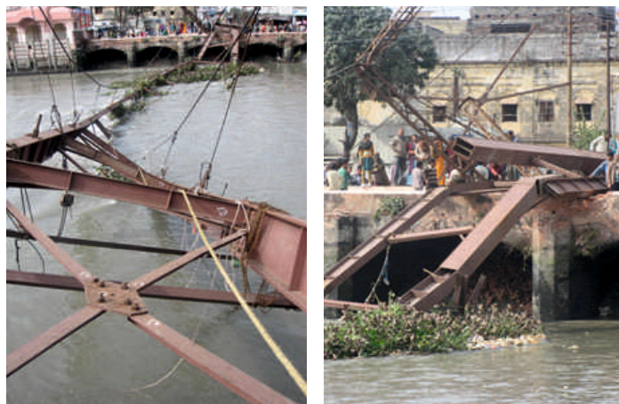
Collapse of 70 m pedestrian steel bridge during erection over Ganga canal at Roorkee
