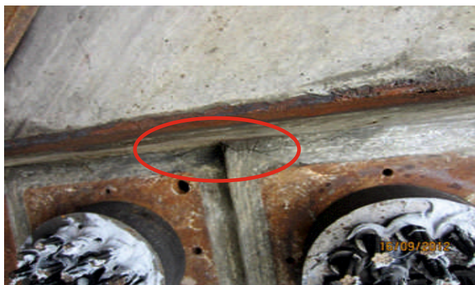
Failure of PSC Box girder as shown in red circle just after transfer of prestress
