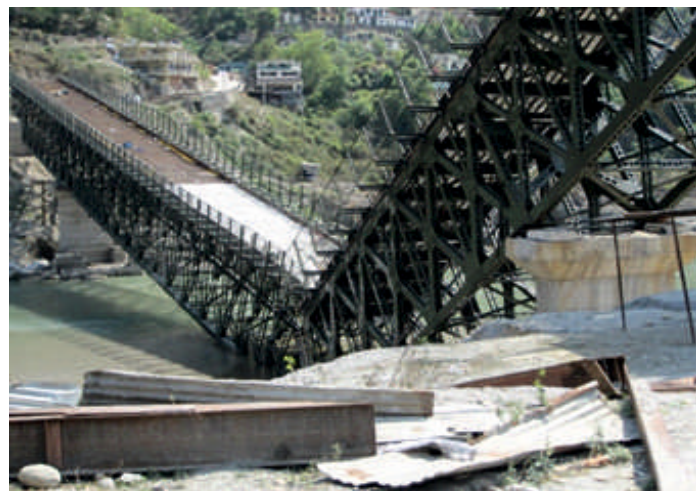
Collapse of 190 m steel bridge with overhangs during laying of pavement at Srinagar, Garhwal
