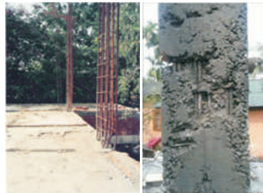
Fig.1 (a) RC columns with kinked rebars, (b) Honeycombing in RC columns
